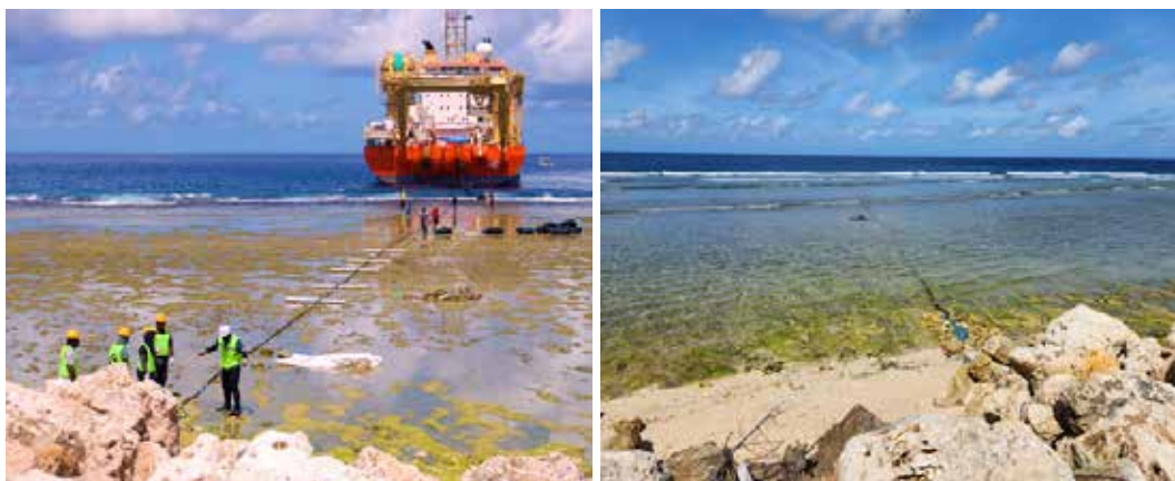
Figure 28: Images of East Micronesia Cable landing into Nauru
